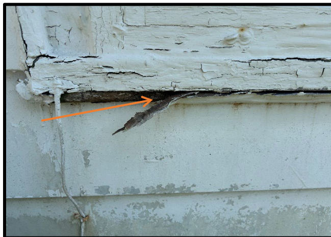
Photo #: 14 Material #: 14 Non-ACM Subject: View of white exterior window caulking, located in FS-3.
