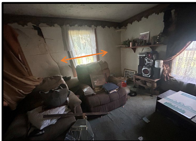
Photo #:4 Material #:4 Non-ACM Subject: View of textured plaster walls, located in FS-1.
