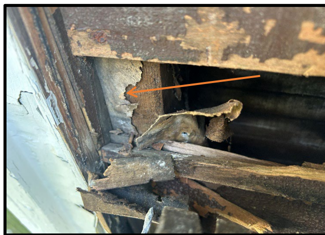
Photo #: 16 Material #: 16 Non-ACM Subject: View of tan exterior wall vapor barrier, located in FS-3.
