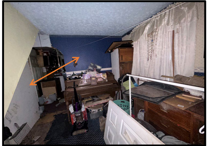
Photo #: 8 Material #: 8 Non-ACM Subject: View of drywall with joint compound, located in FS-1.
