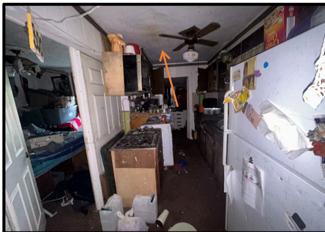
Photo #:2 Material #: 2 Non-ACM Subject: View of smooth plaster ceiling, located in FS-1.
