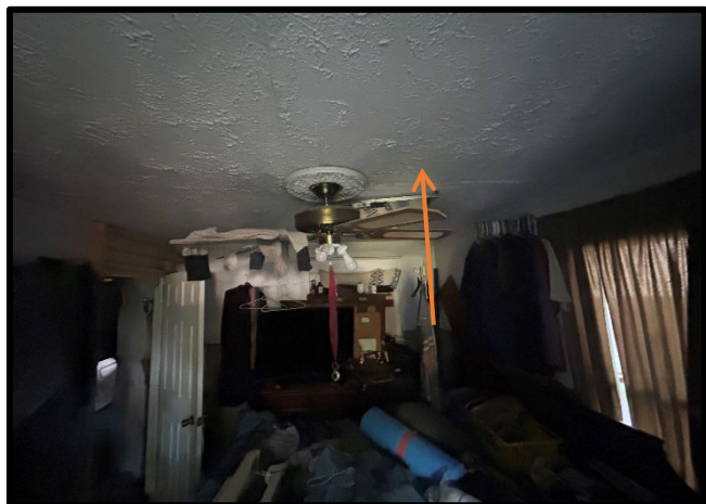
Photo #: 1 Material #: 1 Non-ACM Subject: View of stumped textured plaster ceiling, located in FS-1.
