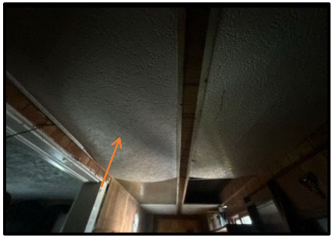
Photo #: 10 Material #: 10 Non-ACM Subject: View of 2'X4' suspended ceiling tile with gouges, located in FS-1.
